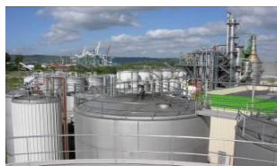
CHP plants - Saipol, France
