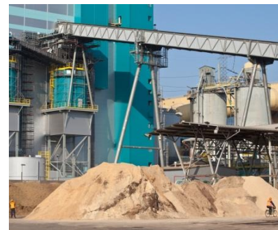
Biomass plant, Polaniec, Poland
