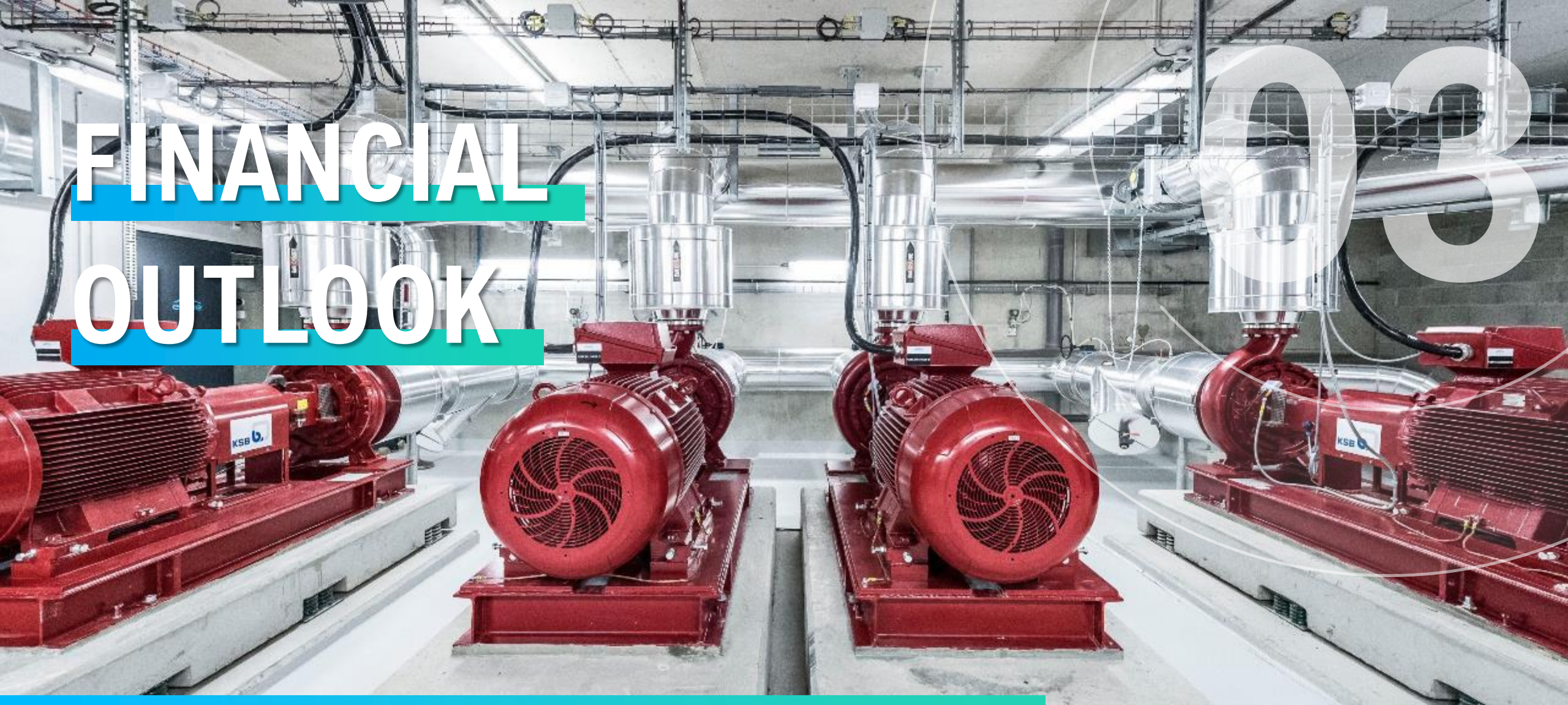
Pumps hot water distribution, The "Thassalia" marine geothermal plant Marseille 13
