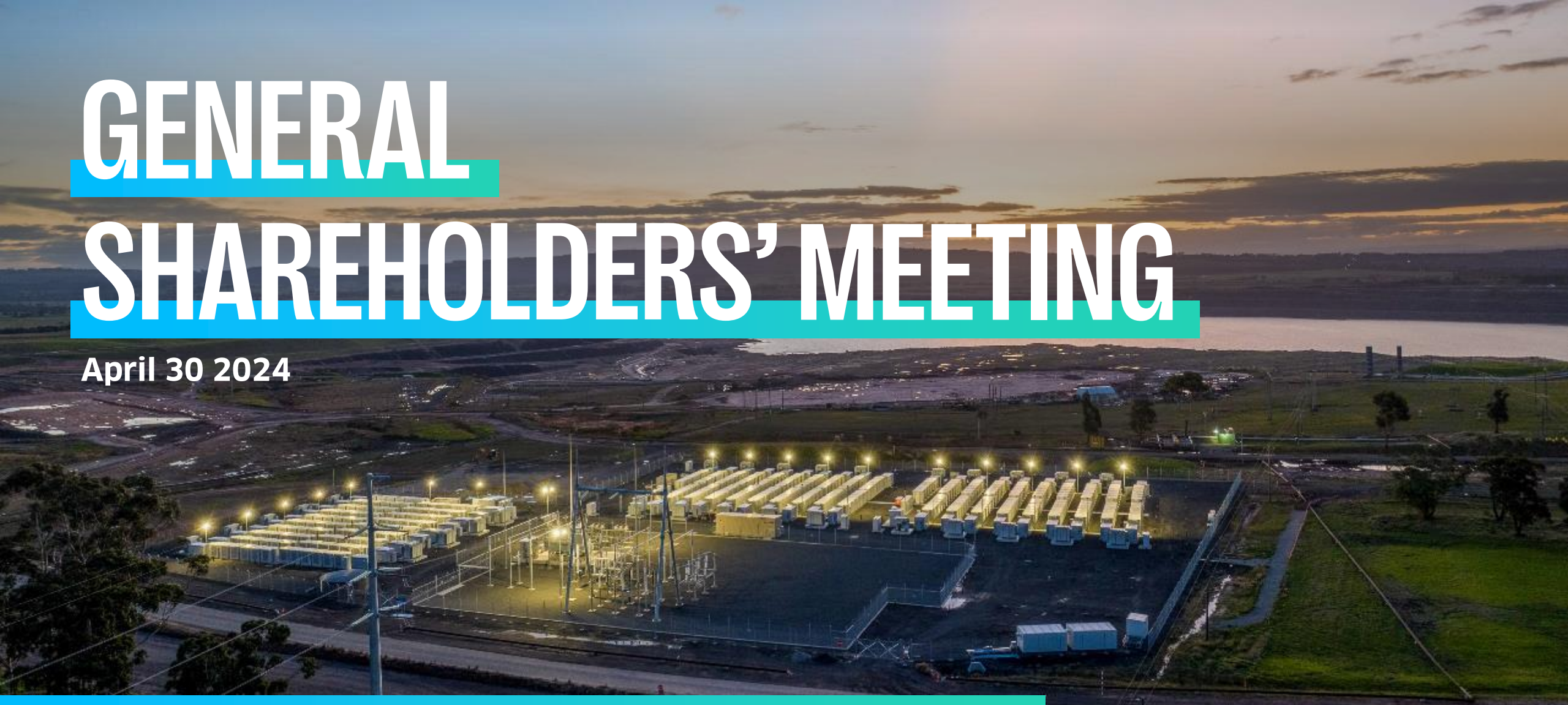
Hazelwood battery energy storage system - Australia
