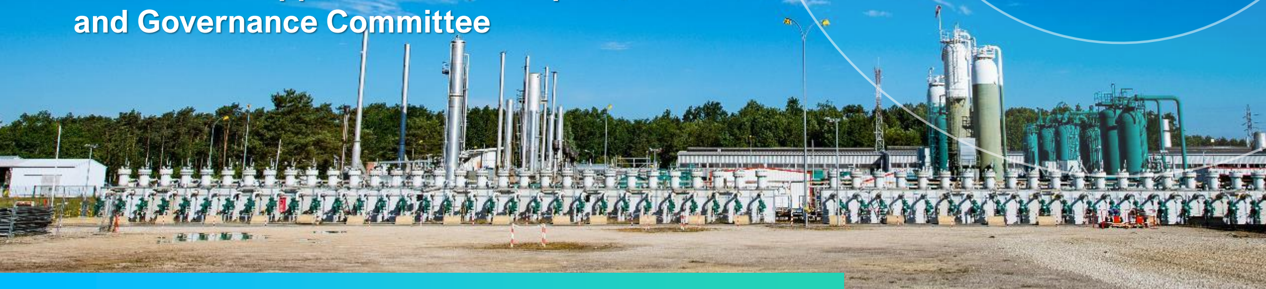
Storengy's Chémery underground natural gas storage facility - France
