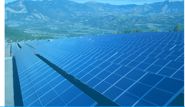
Photovoltaic power plant - Ourbans, France
