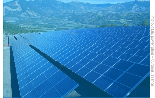
Photovoltaic power plant – Curbans, France
