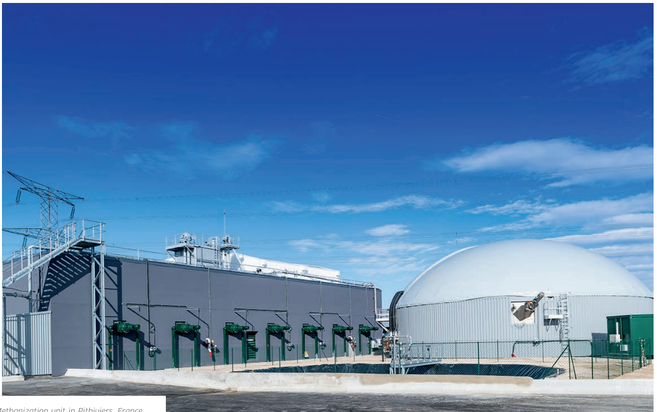
Methanization unit in Pithiviers, France
