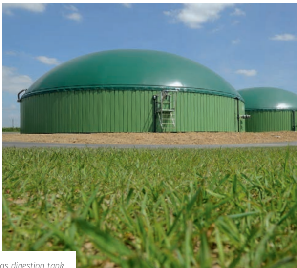
Biogas digestion tank
