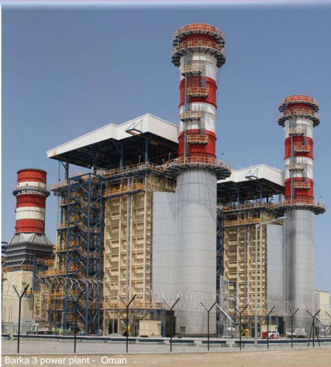
Barka 3 power plant - Oman
